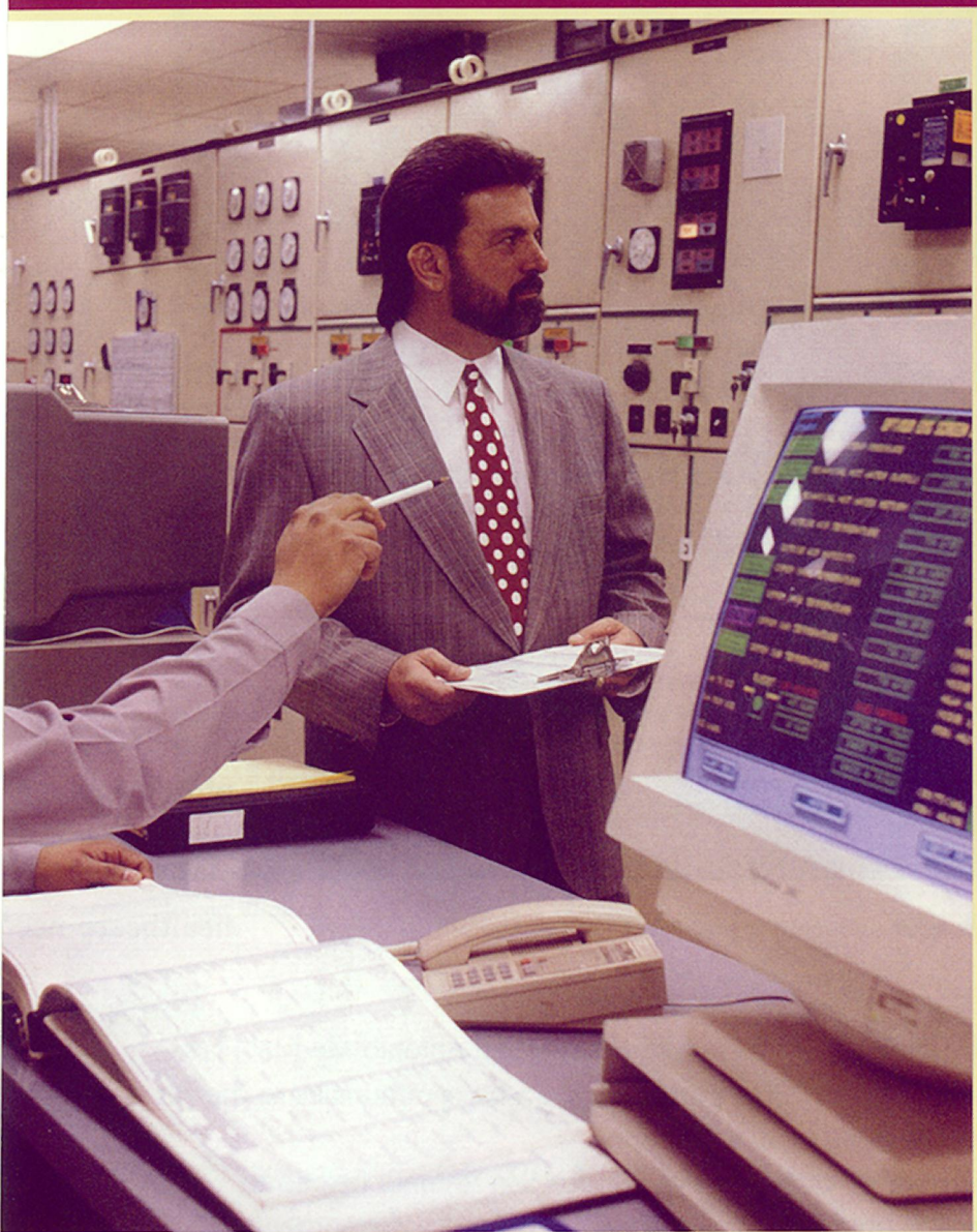
Bill Persi (standing), director of facilities, and Larry Bustos, plant supervisor, monitor the status of the hospital's cogeneration system in 1995.
